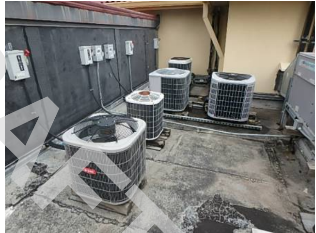
Rooftop condensing units
