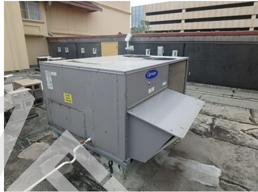
#22 ROOFTOP PACKAGE UNIT
