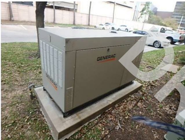
Natural gas-fired emergency generator
