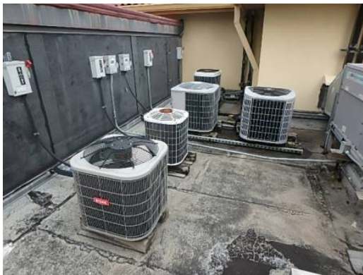
#23 ROOFTOP CONDENSING UNITS
