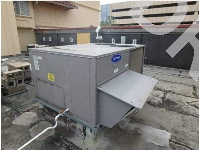
Rooftop package unit
