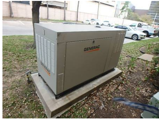
#14 NATURAL GAS-FIRED EMERGENCY GENERATOR
